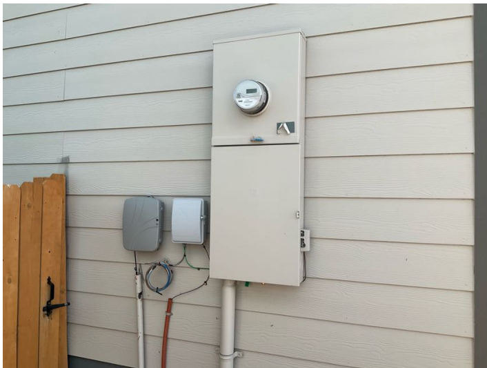
Square D Electricl Panel
