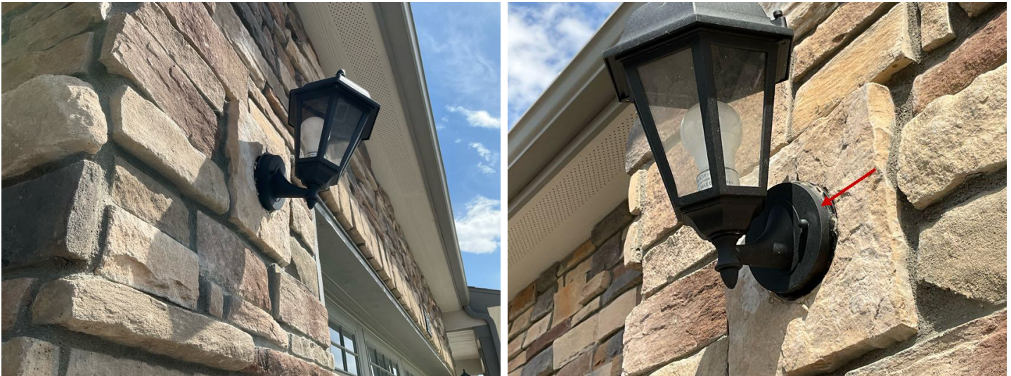
Garage exterior light loose from siding.
