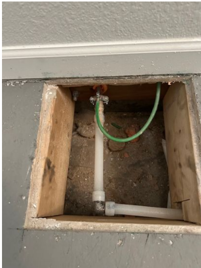
Main water coming into house, through stairway with 5 ft or more to shutoff valve. Where can water be turned off before the house?
