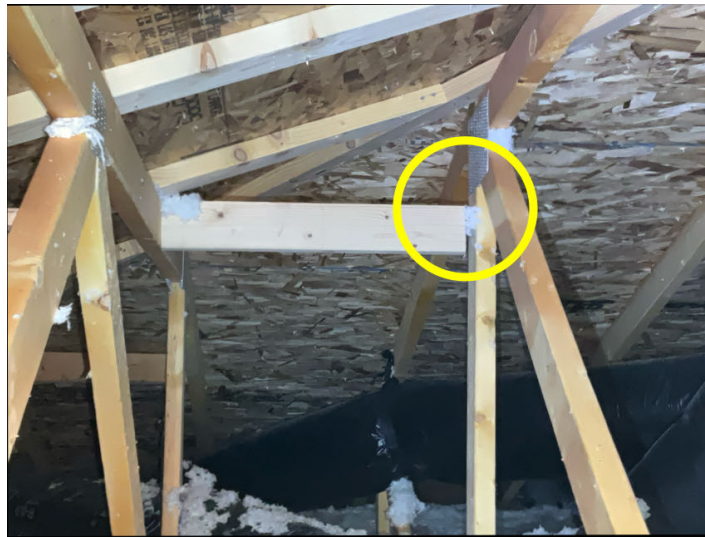
Support board not fully attached.
