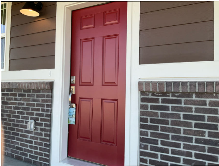
No major system safety or function concerns noted at time of inspection.
