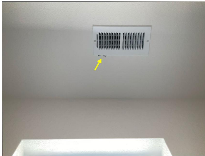
Master bedroom closet bad cut around the vent
