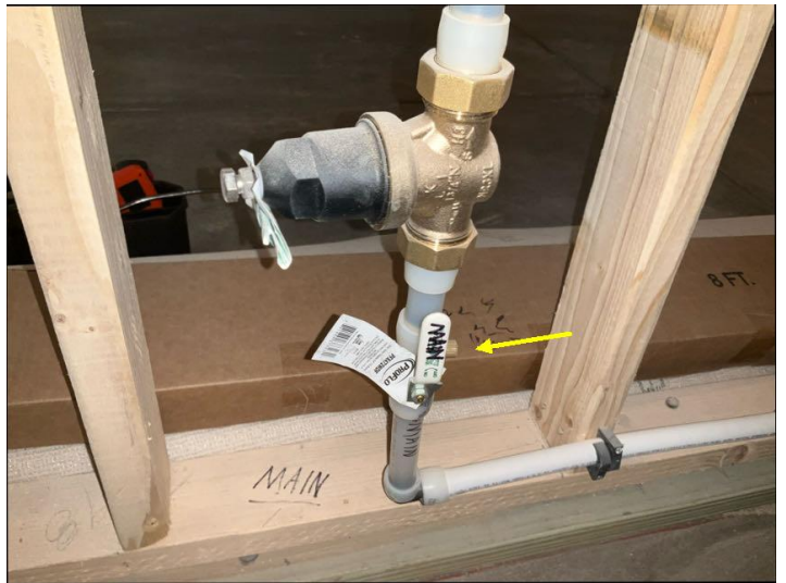
Main water shutoff.
