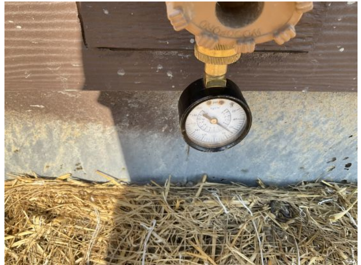
Water pressure is at 70 psi.
