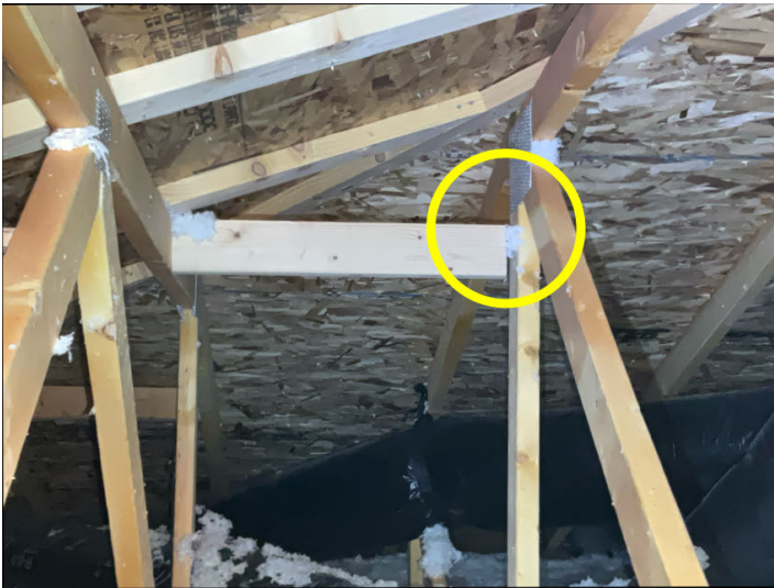
Support board not fully attached.
