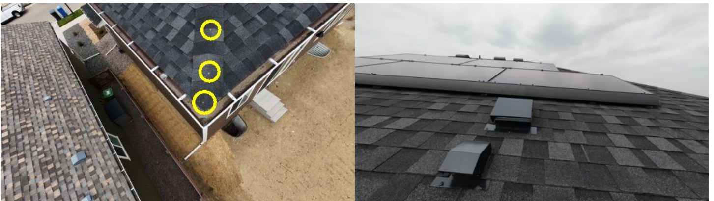
Possible nail heads are visible on the roof surface. Exposed fasteners should be properly sealed to help prevent moisture intrusion and deterioration.
