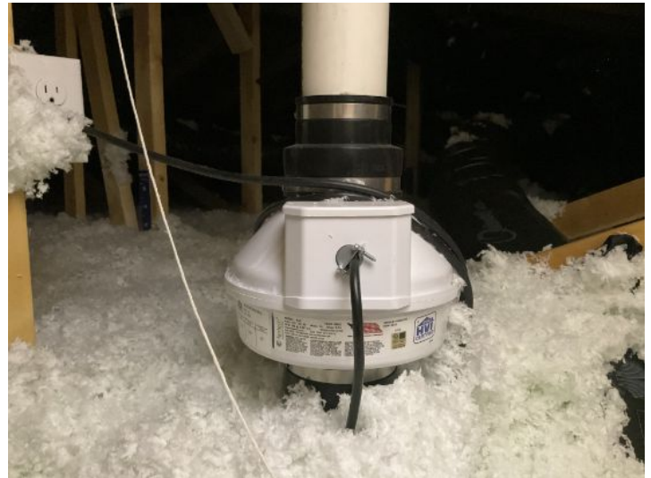
Active radon mitigation system in attic.
