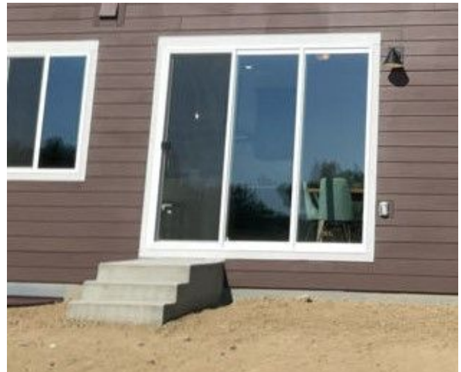
No major system safety or function concerns noted at time of inspection.
