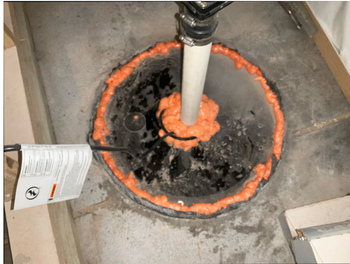
No major system safety or function concerns noted at time of inspection.
