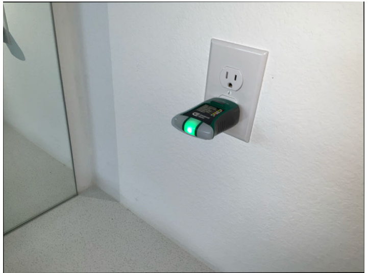
GFCI trip reset is in 1/2 bath on main floor.
