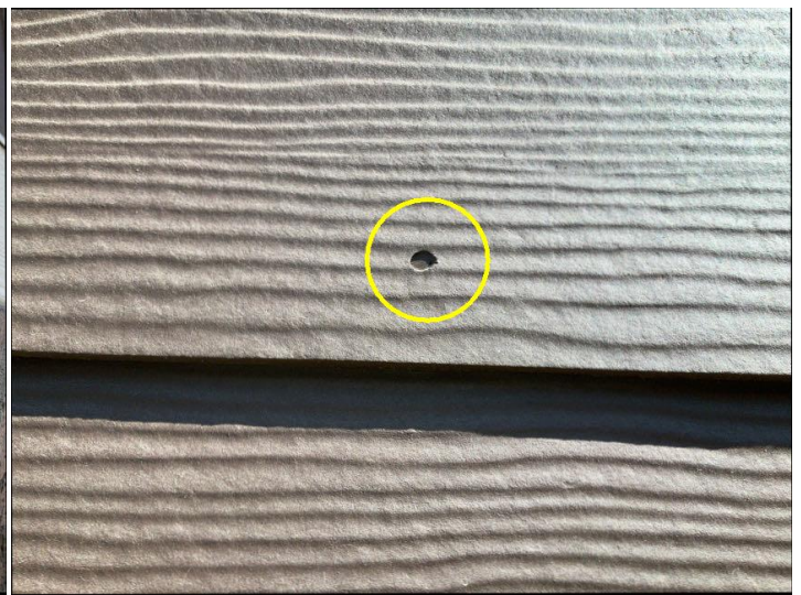
Some siding nails are protruding through the siding. This condition can allow moisture intrusion, damage to the siding material, and reduce the overall effectiveness of the exterior cladding. Recommend repair or adjustment by qualified contractor to help maintain siding, integrity and weather resistance.
