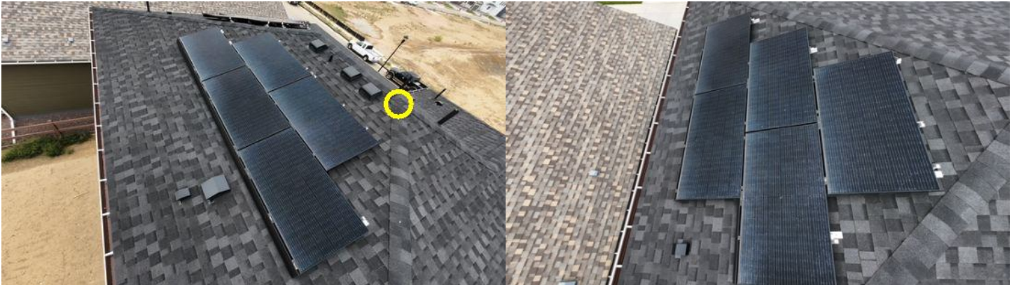
Possible nail heads are visible on the roof surface. Exposed fasteners should be properly sealed to help prevent moisture intrusion and deterioration.
