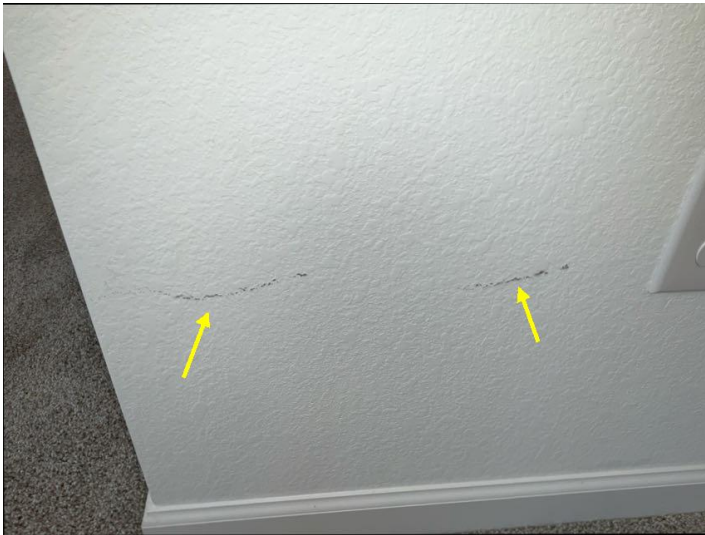
Damage at upstairs going into the loft area.
