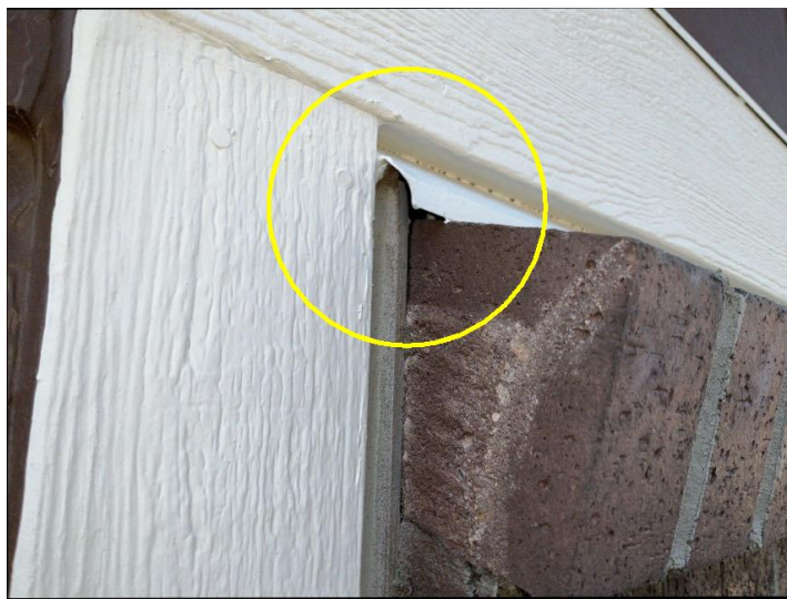
Caulk and seal all gaps, cracks and openings. Left side of house just past front porch.
