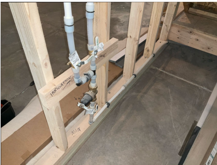
Water shutoffs under stairs.
