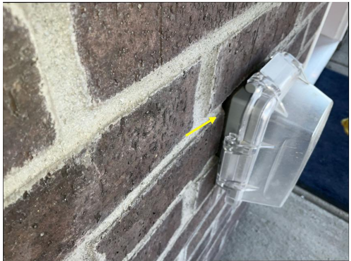
Front porch outlet - Caulk and seal all gaps, cracks and openings.
