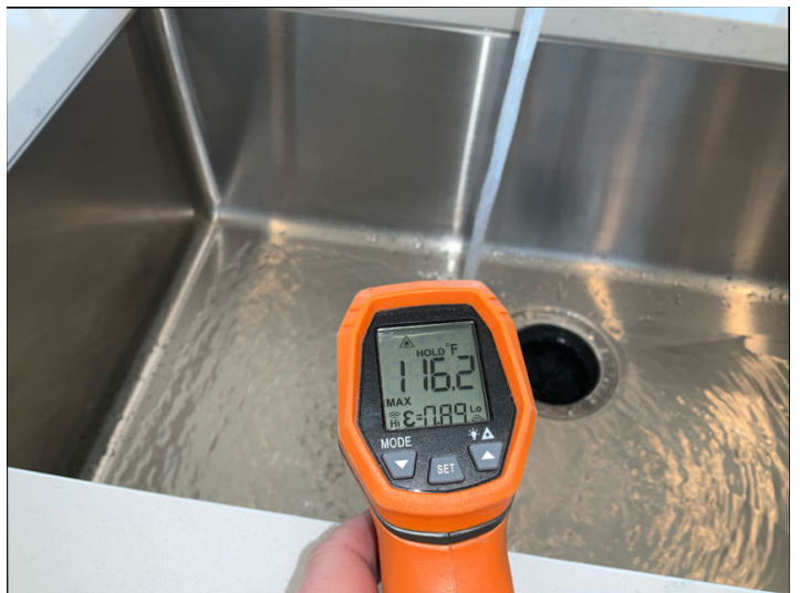
The Highest water temp recorded at the time of inspection.
